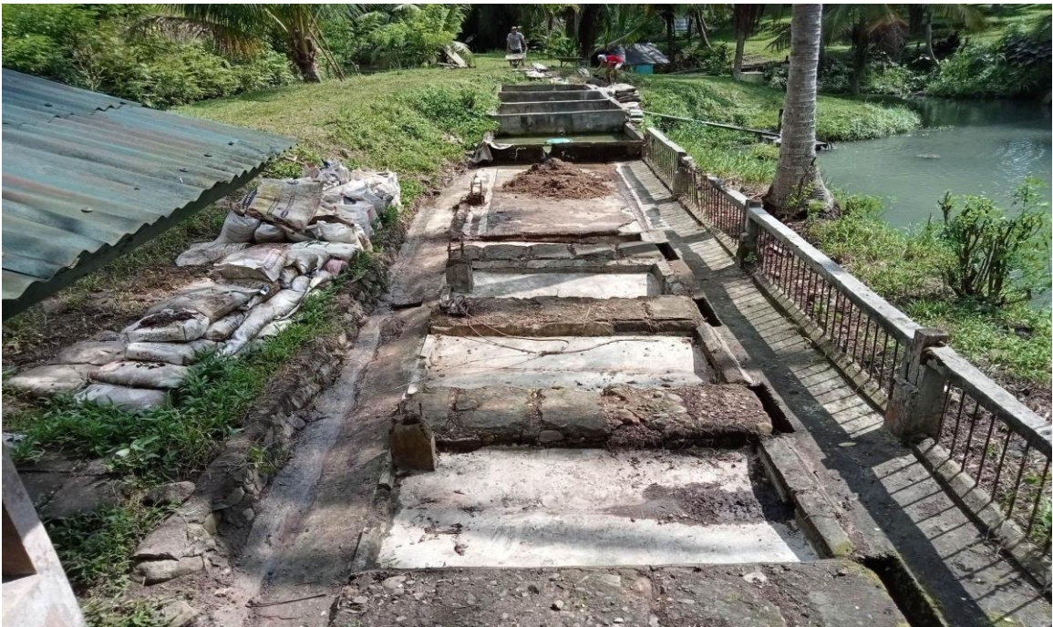
Pathways that need repair
